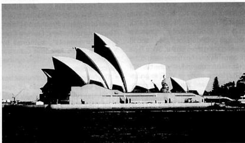
WJE has carried out tests on concrete cores extracted from the shell roof of the Sydney Opera House.
