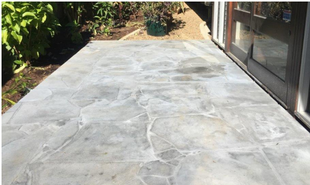
Patio before grout haze cleaning and sealing
